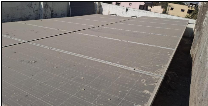
Figure 21 Solar plates at the roof top of a school
