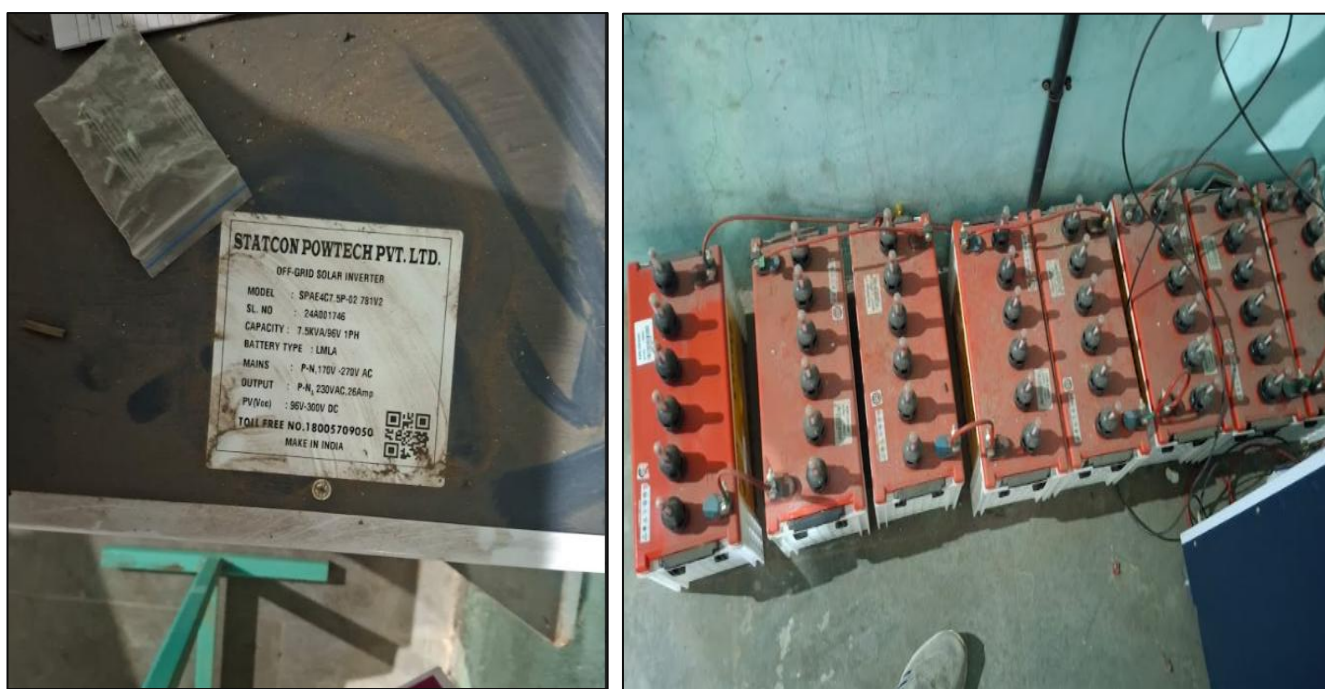
Figure 13 Off Grid Solar Panel Inverter (on the left) and Stored Inverter Batteries (on the right)
