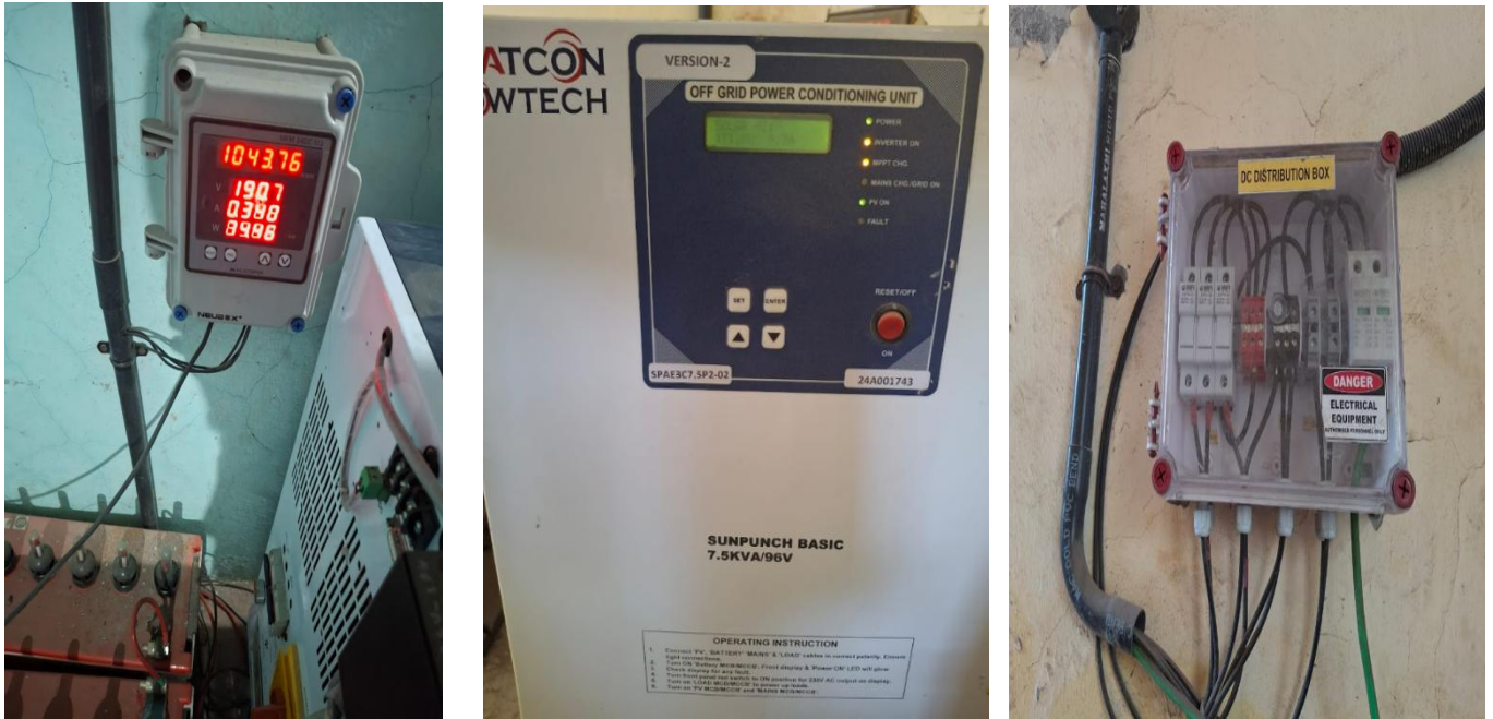
Figure 16 (1) Electricity meter box (2) Off-grid solar inverter (3) Meter box of solar panel
